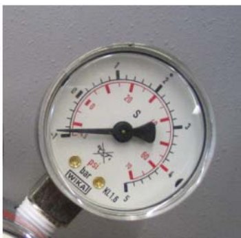
Figure 39 Pressure gauge (low pressure stage) indicating about -0.8 bar (below ambient)
