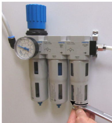
Figure 7. Nitrogen generator gas filter housing removal
