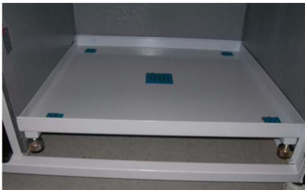
Figure 9 Installed pump tray
