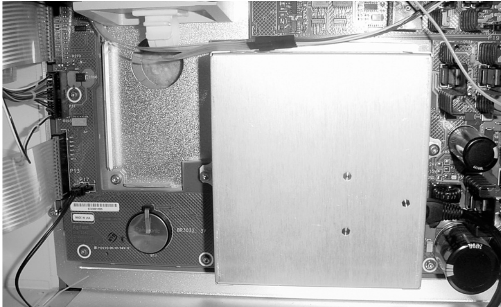
Figure 6 New MIO cover and LAN board assembly installed
